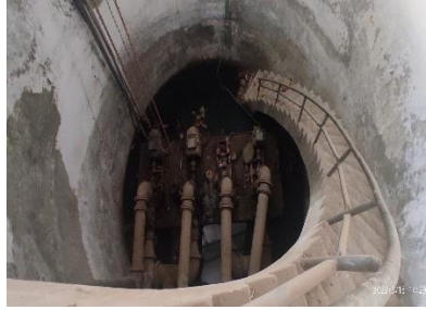
A view of drywell at nawaz sharif disposal station
