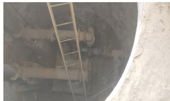
A view of dry well at Zeeshan colony disposal station
