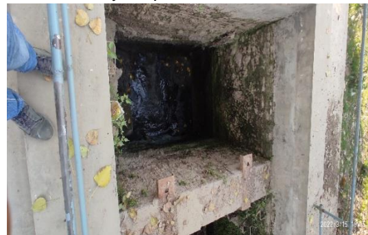
A view of force main discharging into sullage carrier
