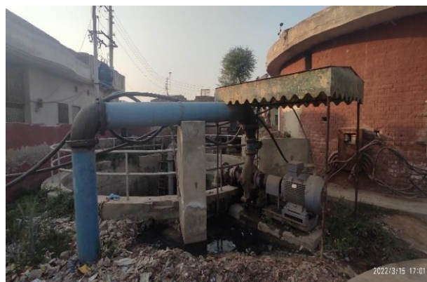
A view of sewage pumping through Force main to sullage carrier
