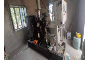
A view of generator installed at nawaz sharif disposal station
