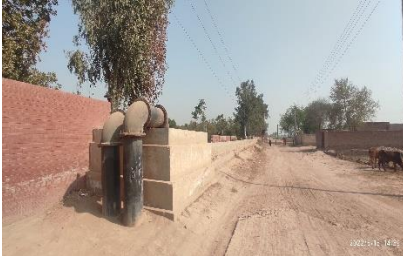
A view of force main (size 24 inches) emanating from nawaz sharif disposal station
