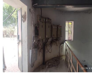
A view of mcc unit installed at nawaz sharif disposal station
