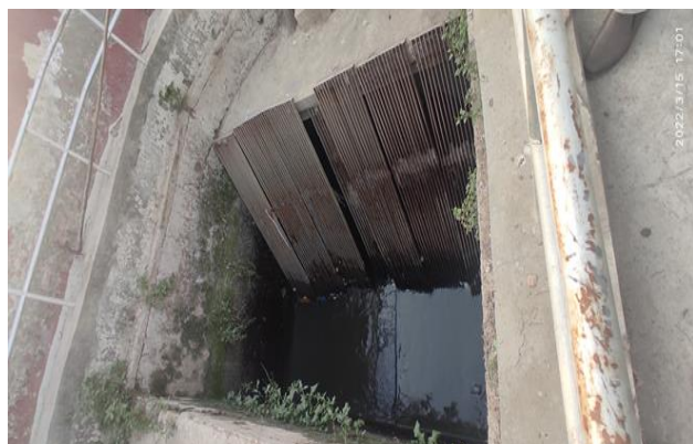
A view of screening chamber at Chungi no. 6 disposal station
