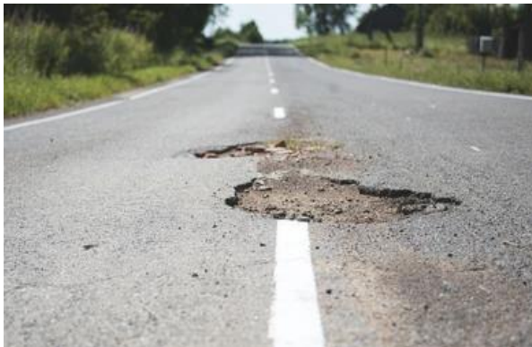
Figure 6: Potholes on the road
