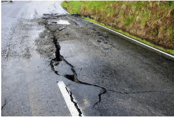
Figure 8: Cracks on the Road
