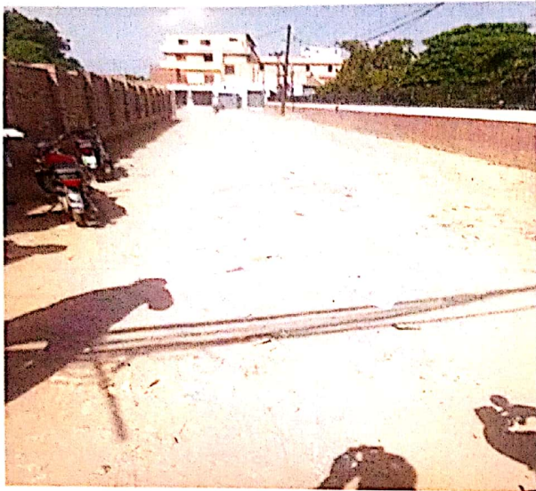
Poor Road near Fazil Dewan Park
